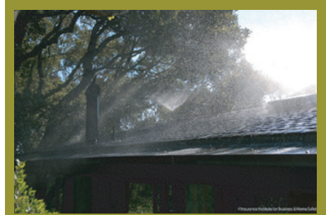
Photo 1. Roof mounted sprinkler.
