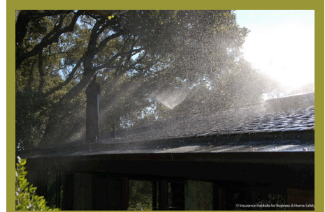
Photo 1. Roof mounted sprinkler.
