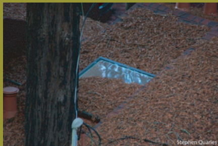
Photo 1. Accumulation of vegetative debris on top of a glass-type skylight on a low-slope roof.
